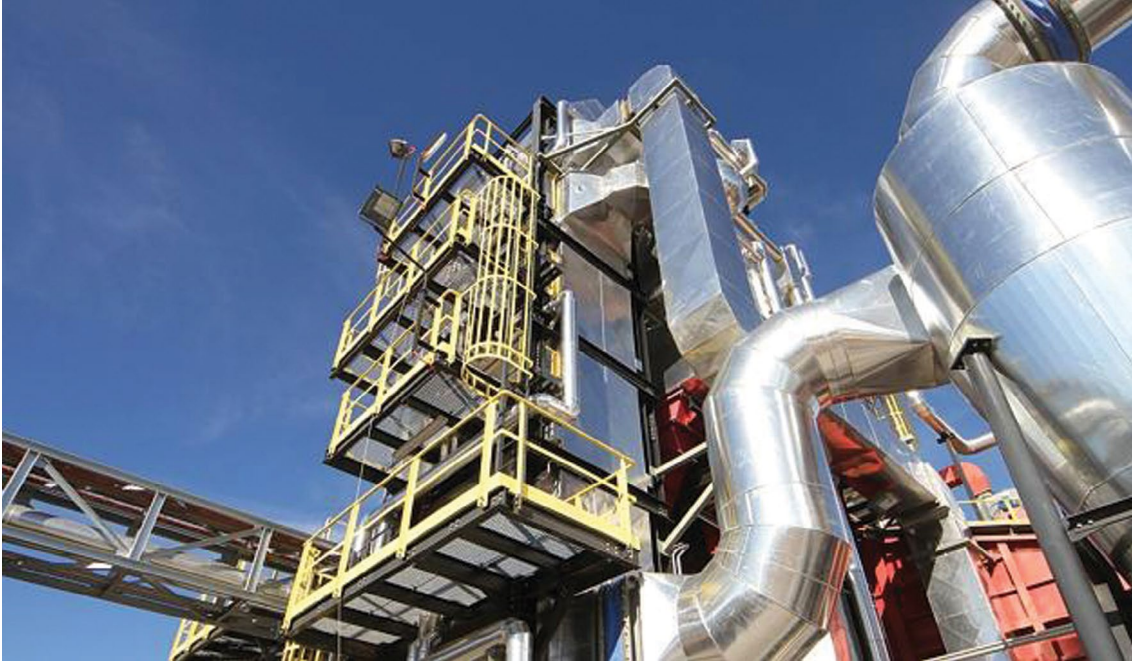
Figure 5. Biomass boiler – full case study see page 39. Photo: Australian Tartaric Products
