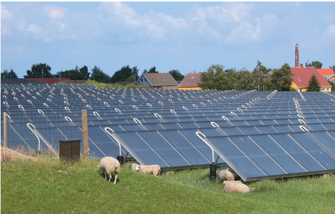
Figure 6. Solar flat-plate collector field – full case study see page 45. Photo: Erik Christensen
