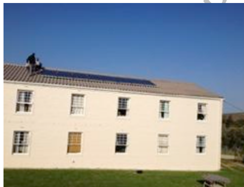
Figure 8: Typical multi family building solar water heater installation, Stellenbosch
