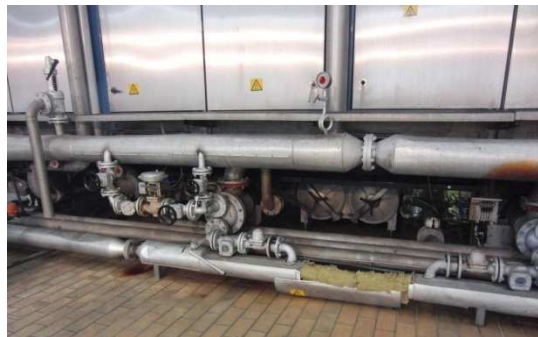
Existing steam heat exchanger
