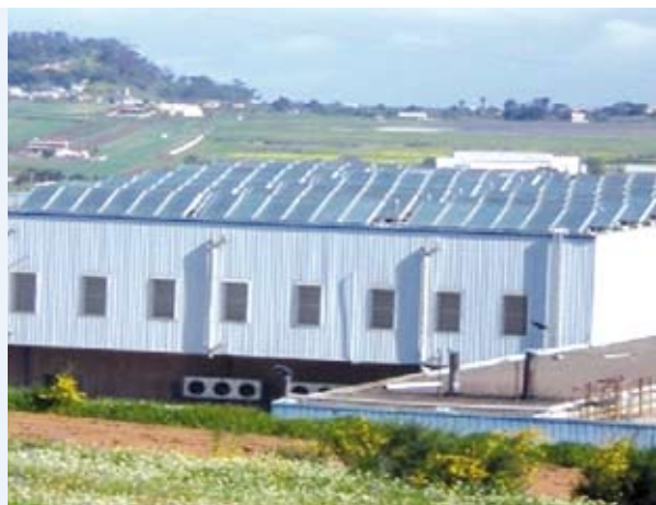
Fig. 1: Flat-plate collectors on the roof of the Montesano production hall, situated on Tenerife, La Esperanza, Spain
