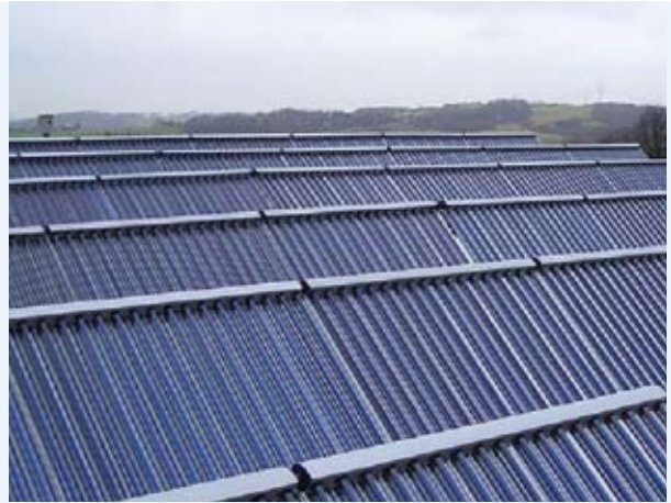
Fig. 3: Vacuum-tube collectors (400 m 2 ) on the roof of Steinbach & Vollmann, situated in Heiligenhaus, Germany
