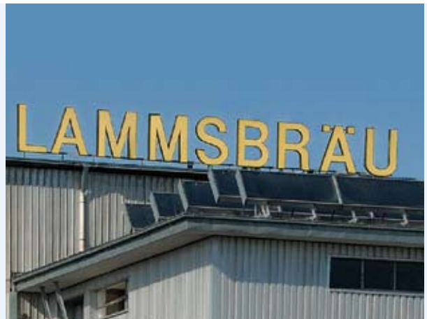
Fig. 4: Flat-plate air collectors on the roof (hot air ventilation pipe on the right hand side)
