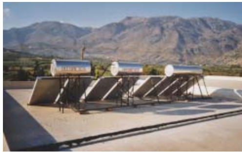
Flat plate collector mono-blocs on a roof in Greece
